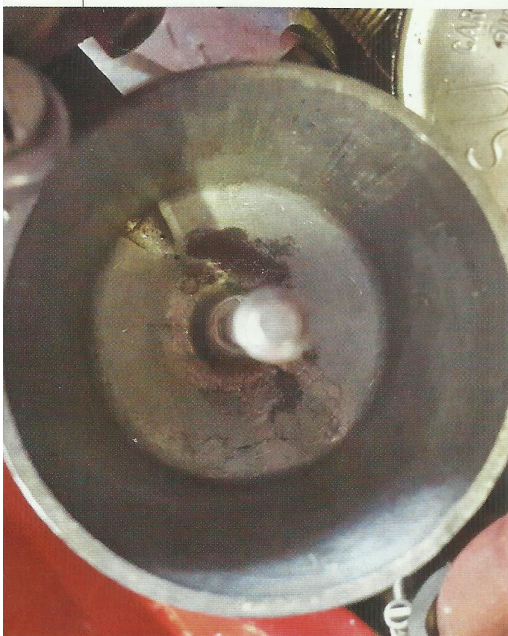
Corrosion in float chamber
